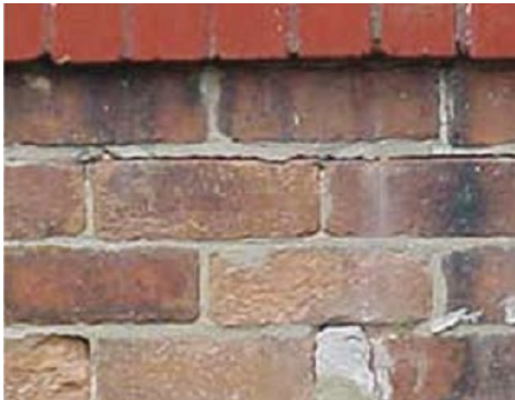
Fig4—Horizontal cracking in mortar joint
