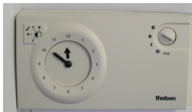
Typical heating time controller
